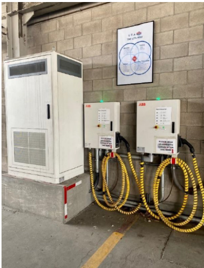
Plug-in charging infrastructure
